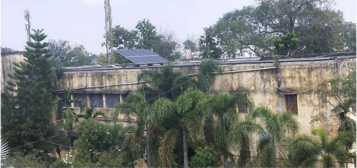
Fig- Solar PV panel system present on the roof of Administrative Block
