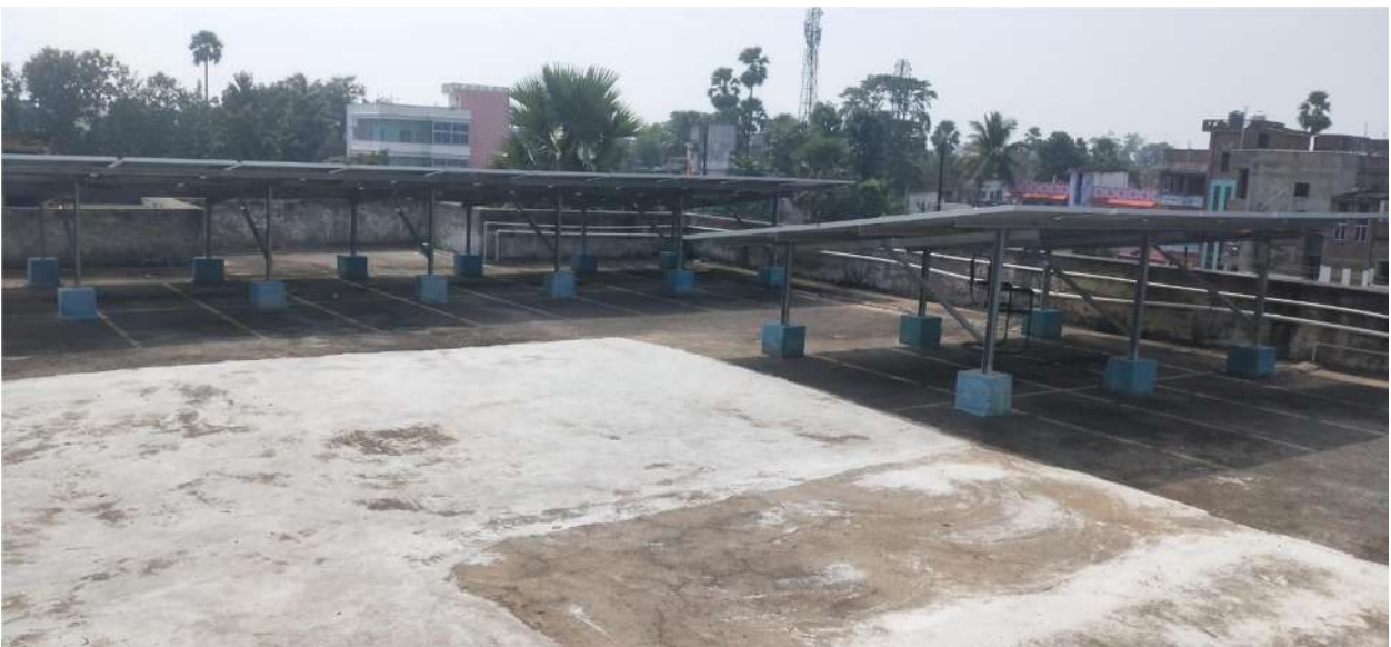
Fig- Solar PV panel system present on the roof of Arts block
